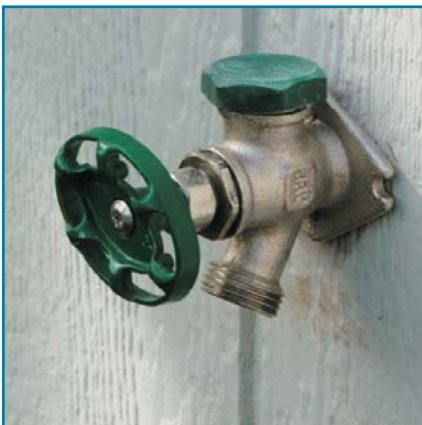
A hose bib with built in anti-siphon backflow protection.
